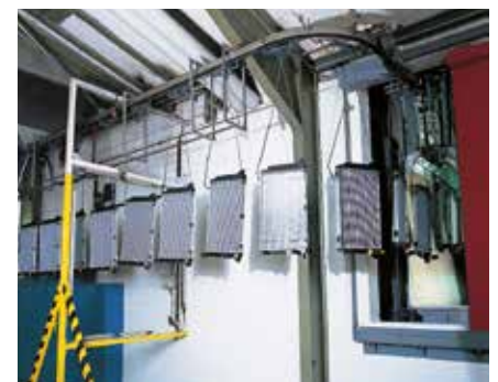
Electrostatic paint line
